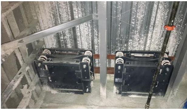
Figure 2 Two TMDs installed underneath the floor system
